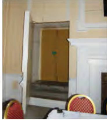
A fire escape to/or from the Finance Block (not for disabled). The Insall/Maggle's scheme will rely on the Hogarth Stairs as a main escape route.
