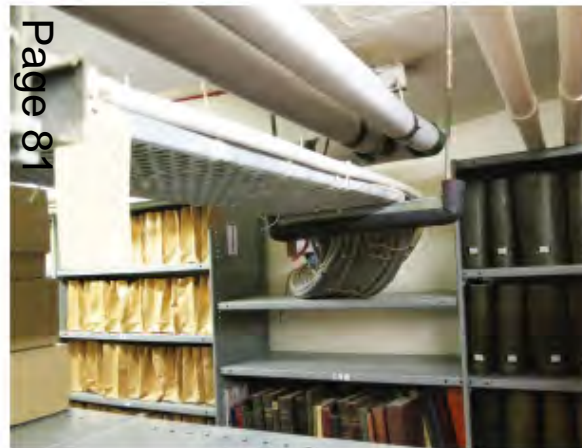
Unconditioned archives in the East end are at risk from exposed overhead services. The existing archives are not improved by the Insall/Maggle's Scheme.
