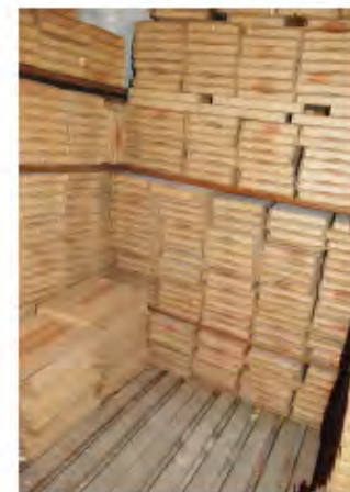
Unconditioned storage areas in the East End. The existing archives are not improved by the Insall/Maggle's Scheme.
